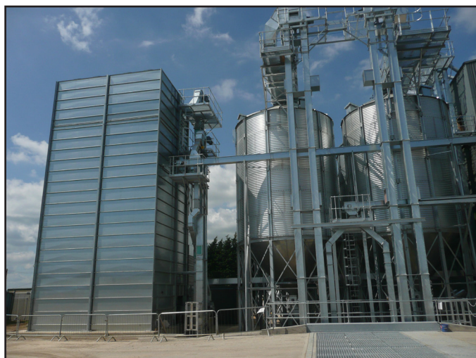
Grain drier and intake system,
