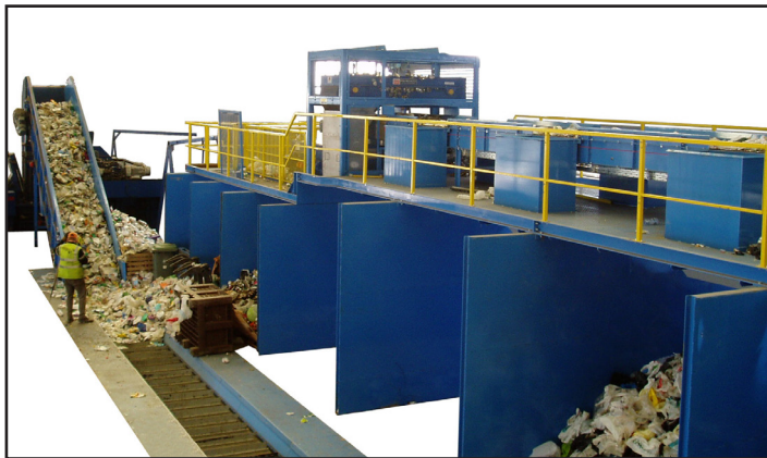
Baler Feed Conveyor.
