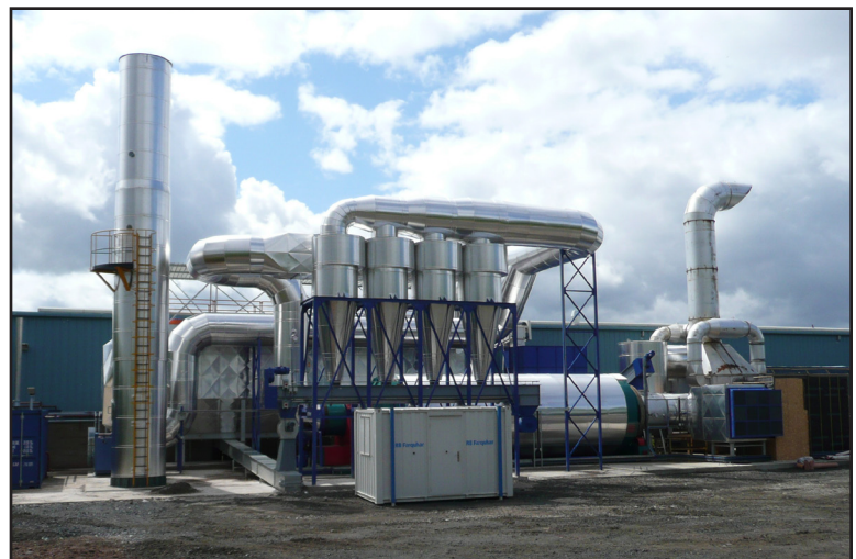
Wood Dryer at Biomass Plant
